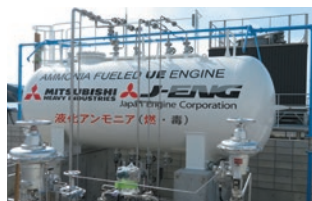
Ammonia fuel tank
