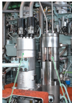
Fuel injection pump (left) Water injection pump (right)
