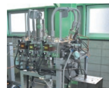
Hydrogen injection unit
